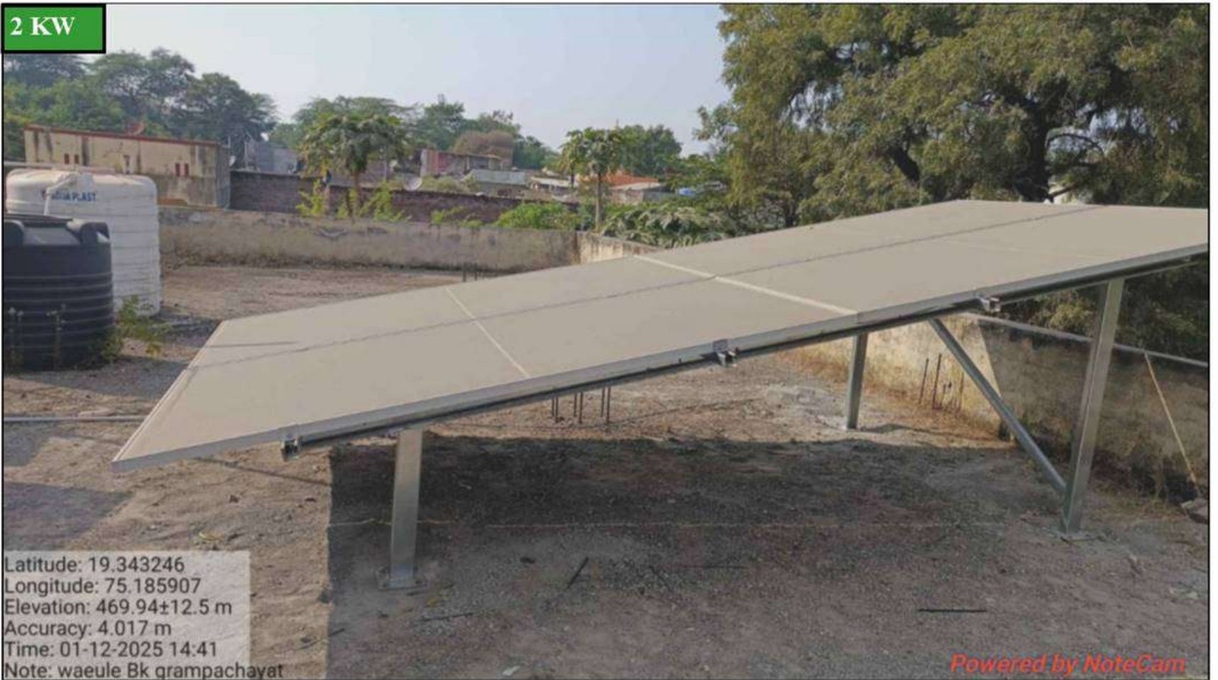
Grampanchayat building - Solar system at village Wadule Bk.
