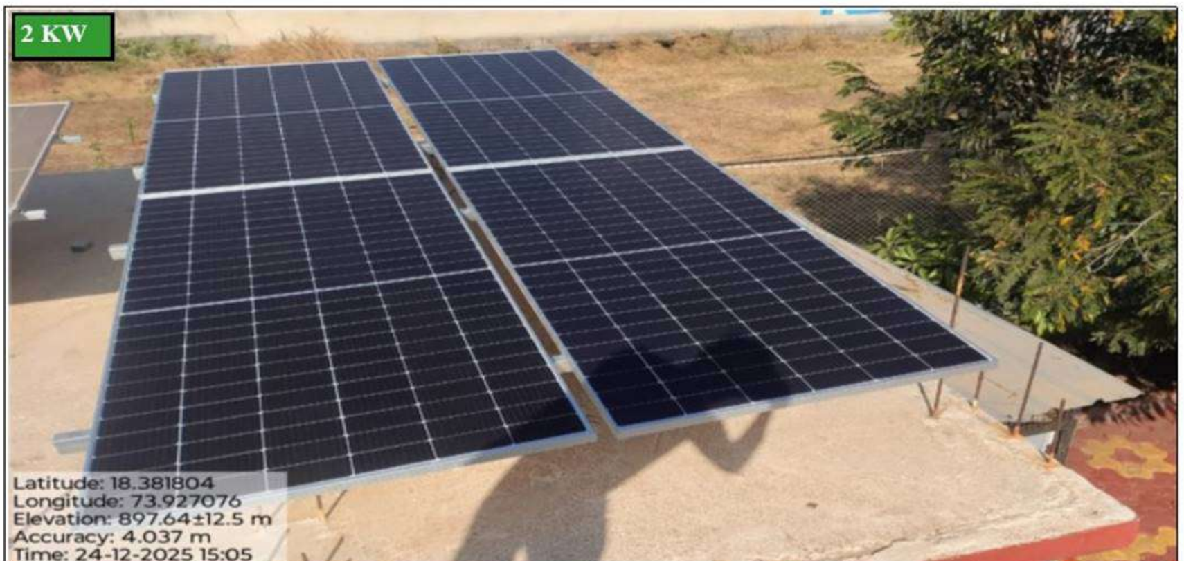
Z P School - Solar system at village Bhivari
