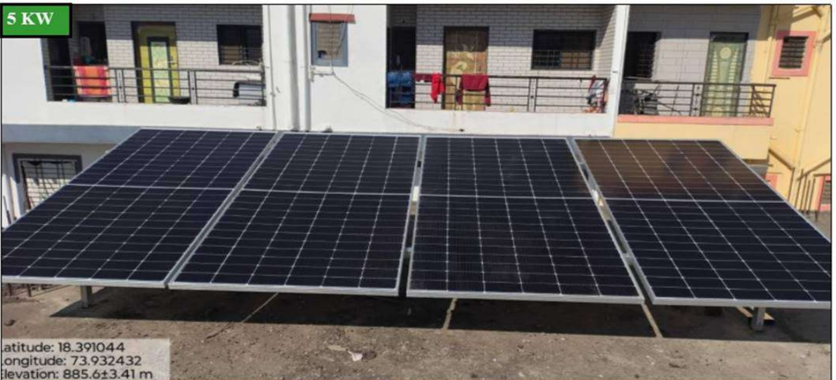
Z P School - Solar system at village Bhivari
